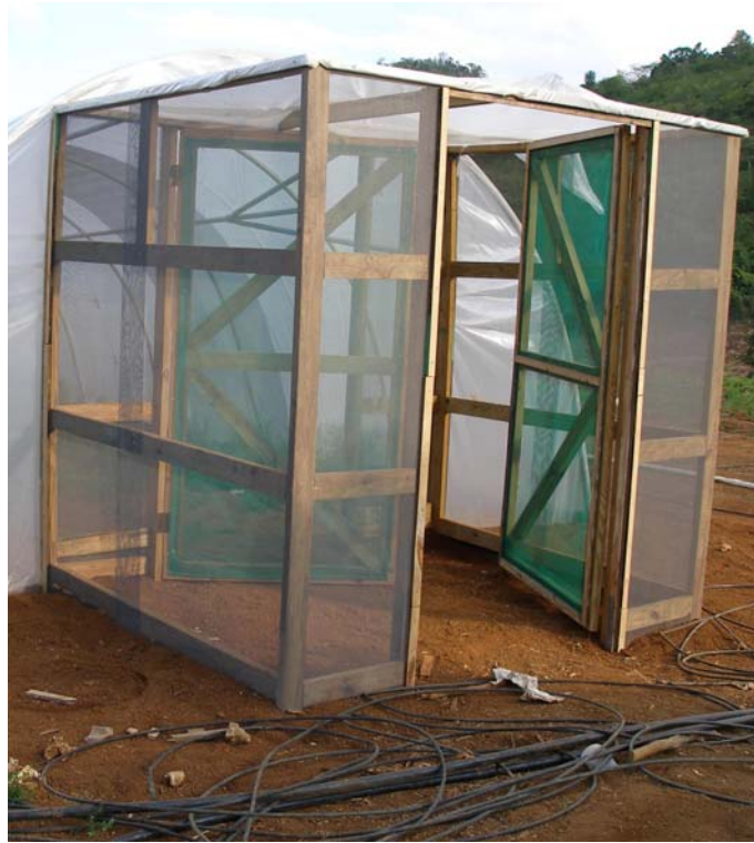
Figure 34 Entrance door protective enclosure
