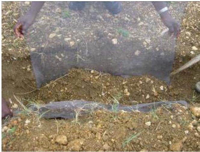
Figure 22: Anchor mesh partially buried in 6 inches of soil
